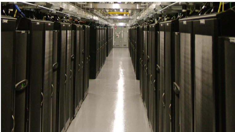
Massachusetts Green High Performance Computing Center (mghpcc.org)
